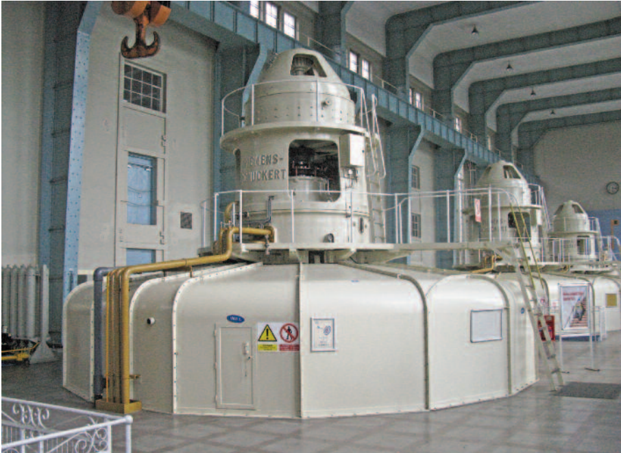
Fig. 8. The three Francis turbines, built by Siemens-Schuckert in 1929, in the Ardacrusha power station, County Clare, Ireland.
