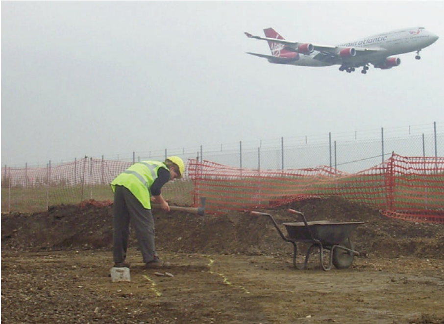
Fig. 4. Heathrow Terminal 5 was one of the biggest construction projects in the world. Excavations by Framework Archaeology in advance of the construction works uncovered almost 9000 years of history. Here, 6000 years separates the cursus , a Neolithic ceremonial way, from the airliner flying above. The excavation took place between two of the busiest runways in the world (copyright of Framework Archaeology, 2011).
